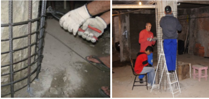
Figure 120: Extension of the useful life of a concrete structure from the 1960s, which houses 42 families in a vertical tenement condominium in downtown São Paulo. (OLIVEIRA et al., in: Annals of 54th Brazilian Concrete Congress). Source: IBRACON, 2012
