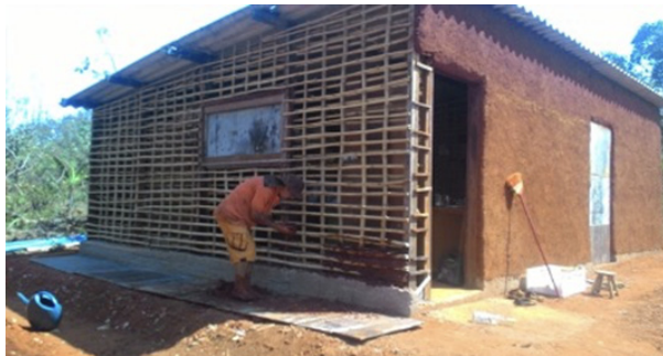
Figures 107, 108 and 109: Pilled up made of Hand Taipa (mud with wood) wall filling. Students of UnB-Planaltina. First taipa (mud with wood) was built on the land ranch. The current house is practically completed. Source: Gustavina Alves da Silva
