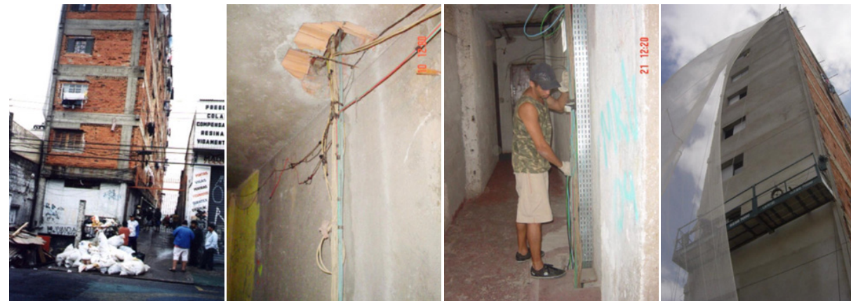
Figure 119: Before, during and after the facade renovation. Source: REHABILITATE PCC US p.
