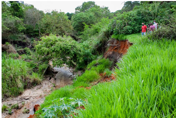
Figure 55: Group of volunteers makes visits to check the situation of the soil erosions. Source: : https://blogsosribeirao.wixsite.com/sosribeirao .
