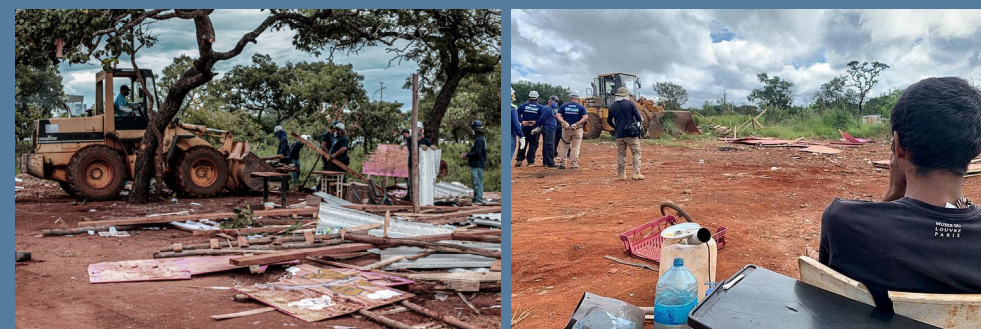
Figure 63: Wreck of houses and school by operation. Photo: Scarlett Rocha
